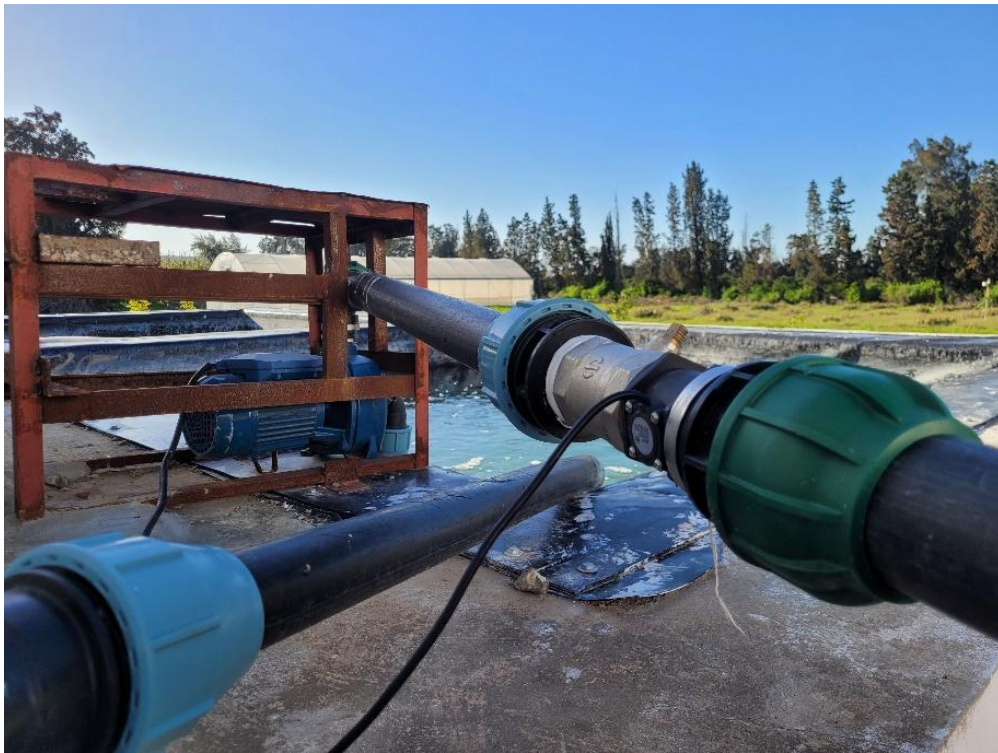
Figure2: Pump and installed flow meter
